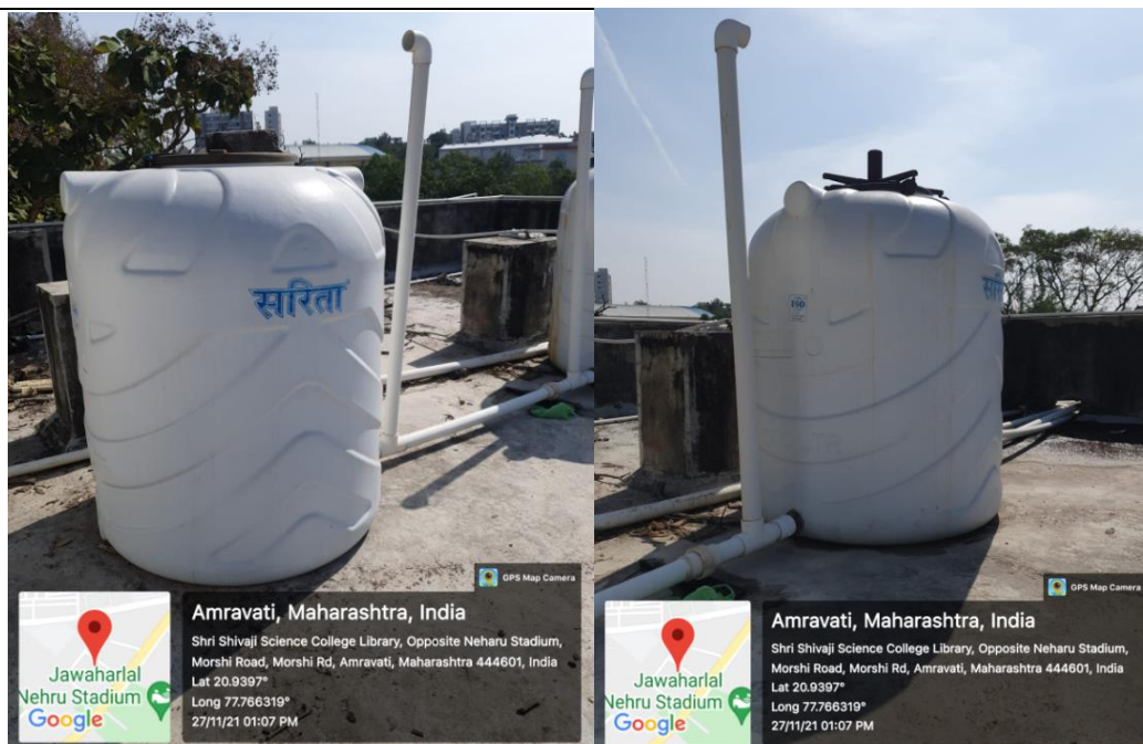
Well-connected pipelines and water tanks are established in the college for proper management of Water Distribution system
