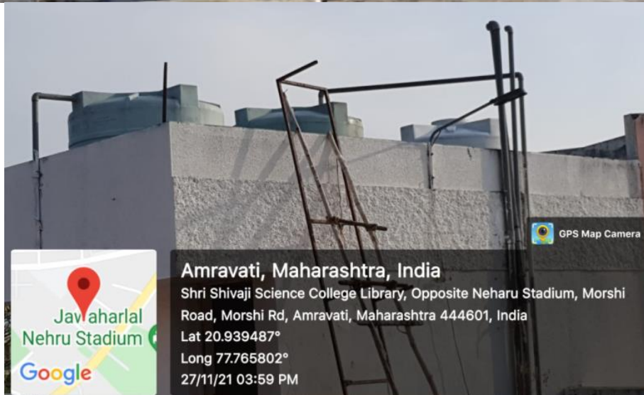
Well-connected pipelines and water tanks are established in the college for proper management of Water Distribution system
