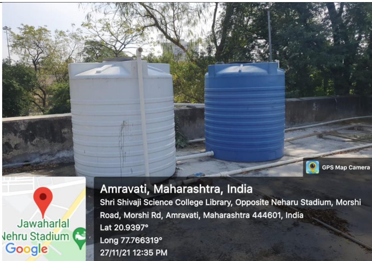
Well-connected pipelines and water tanks are established in the college for proper management of Water Distribution system
