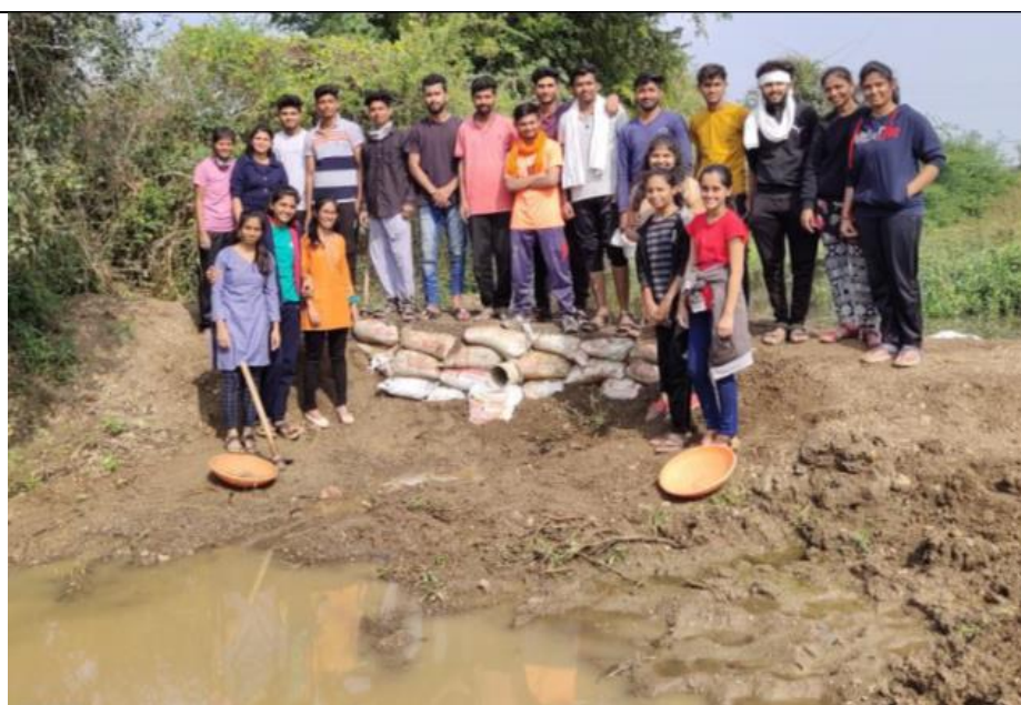
Construction of ENB for increasing groundwater recharge by the NSS students in the NSS Camp of Our college 2019-20
