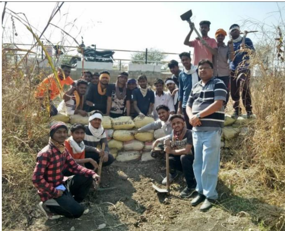
Construction of ENB for increasing groundwater recharge by the NSS students in the NSS Camp of Our college 2018-19
